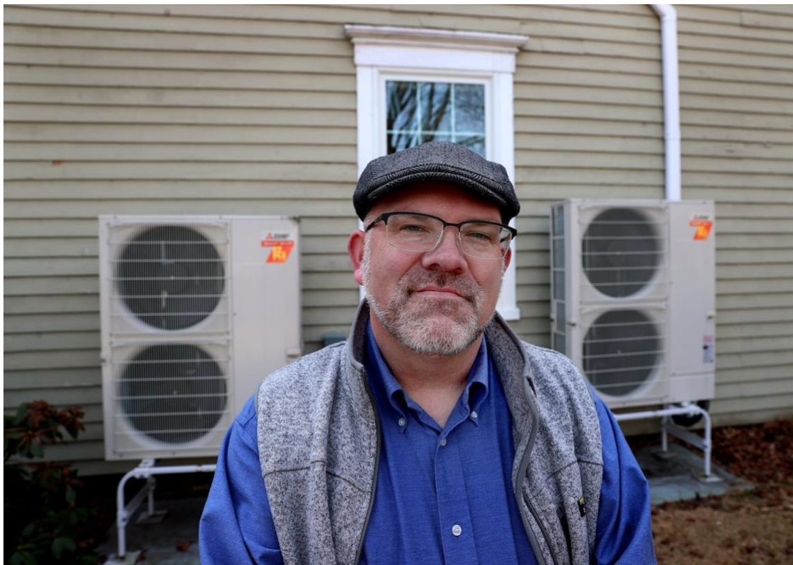
Andrew Feland, near the heat pumps at his home in West Boylston. David L. Ryan/Globe Staff
